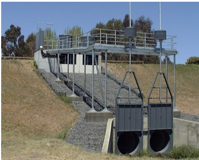
Old Vale Creek stormwater outfall penstocks and flood pumps
